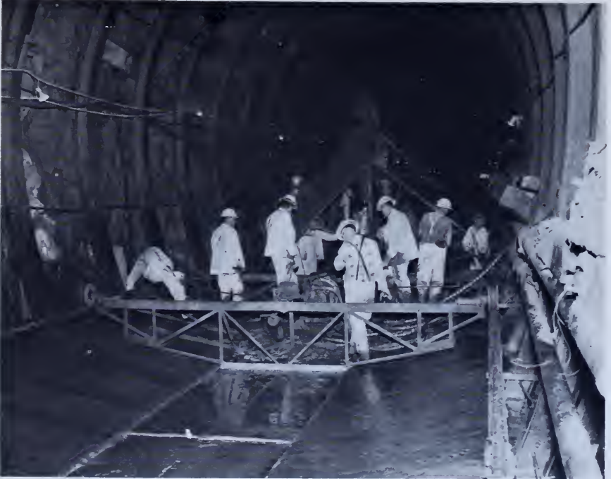
Figure 142. —Placing concrete with slip form in invert section of Spring Creek Tunnel No. 1, Central Valley project, California. P416-229-9608.
